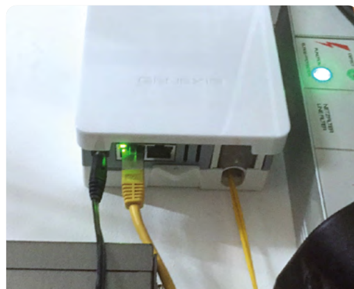
Network terminal device
